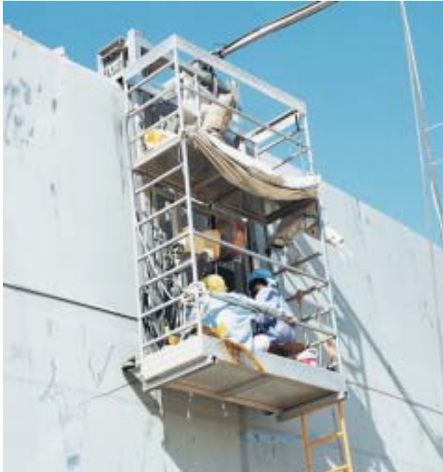
Figure 2. An A2 Circotech machine welding the horizontal joint between the second and third courses.
