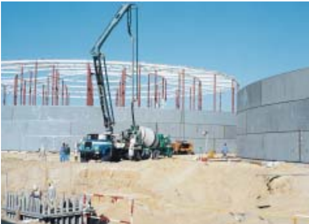
Figure 1. A general view of the site during the early stages of construction which adequately shows the size of the tanks and the number of welded joints involved.
