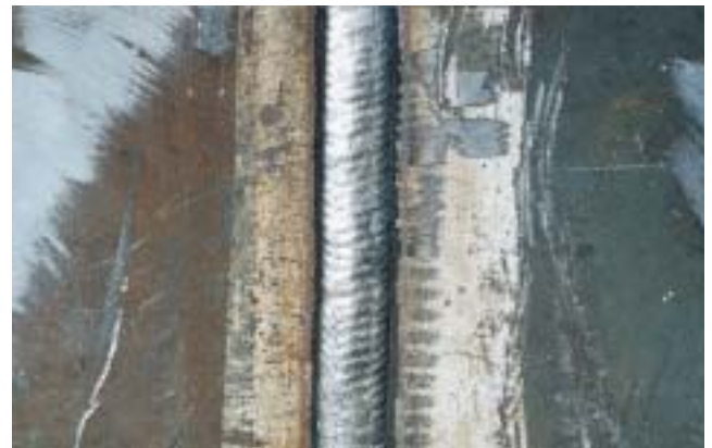
Figure 3. Vertically welded joint showing the flat and smooth profile produced by the Railtrac machine and OK Tubrod 15.14A. The minimal spatter also simplifies preparation for painting.
