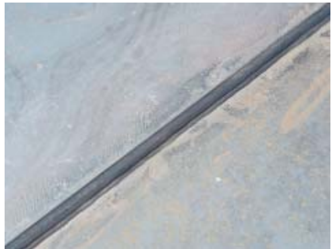
Figure 6. A two-pass lap joint as applied to all floor joints and welded with OK Autrod 12.32 and OK Flux 10.71.
