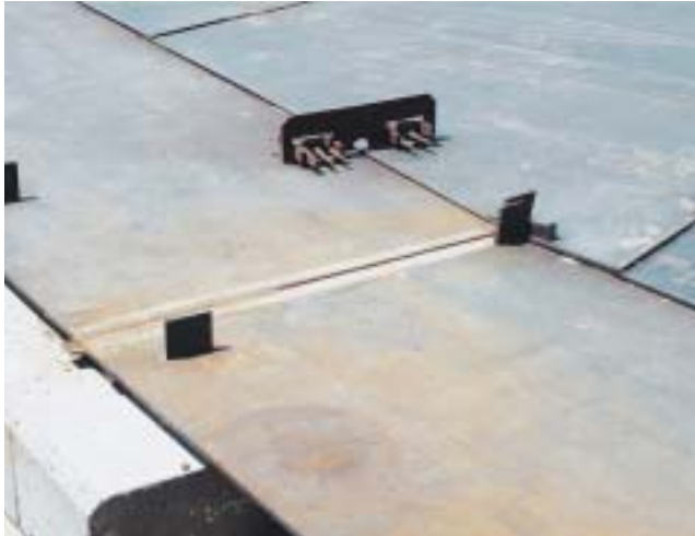
Figure 5. A view of the annular plate segments on which the shell is erected. The fully welded floor can also be seen, but is not welded to the annular plate at this stage.
