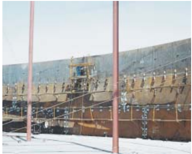
Figure 7. Guy ropes attached to the strong backs which serve to reduce distortion, especially where MMA welding.
