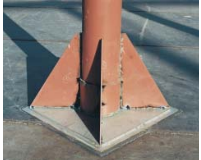
Figure 8. The roof support bases clearly showing the stainless rubbing plates. Corner fences will ultimately be welded to the tank floor to restrict movement to within restricted limits.
